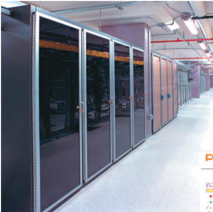
FIGURE 3 Metropolis New Media installs their customers' systems in this Northern California data center.
